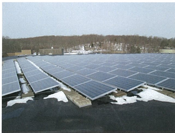
Figure 4.1: Typical ballast mounted solar PV array.
